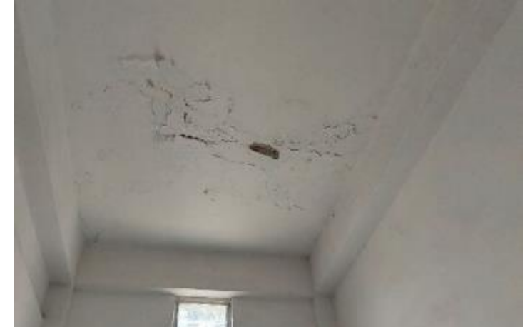
Photo of spalling concrete (Refer to PSI Reports in TCOT)
