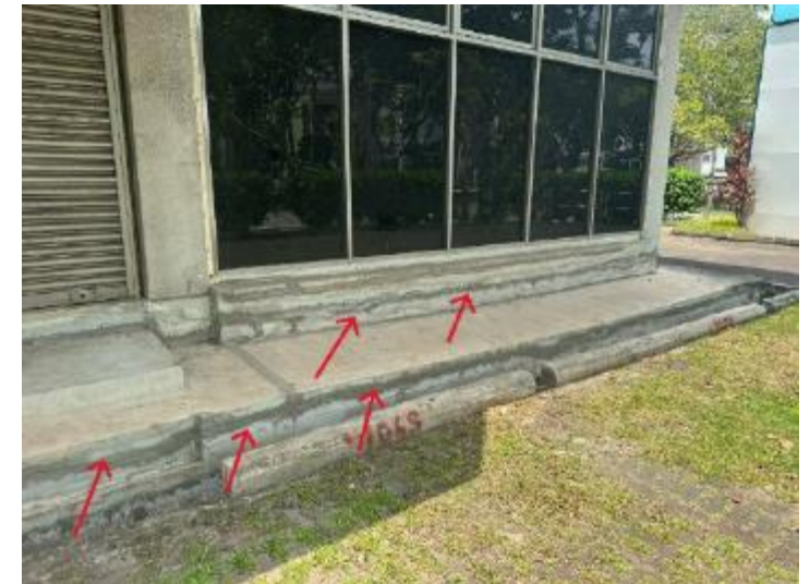
Photo of ground settlement at building apron (Refer to PSI Reports in TCOT)
