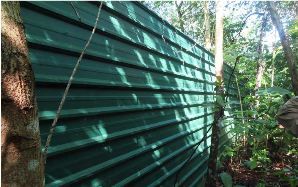
Figure 5.10 Hoarded built-up area of the Jurong Region Line Integrated Rail & Bus Depot.
