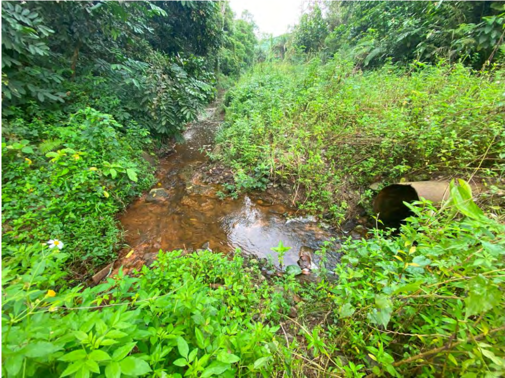
Figure 8.20 Example of a subsurface culvert channelling stream flow from sampling point A2 to the junction where A2, A11 and A12 intersect (Figure 8.21) .
